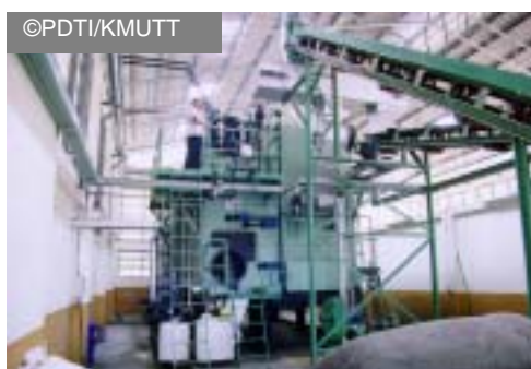
©PDTI/KMUTT Fluidized-bed boiler for superheated steam production, Thailand
